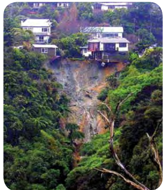
Large landslide in Kelson, Lower Hutt (2006).
