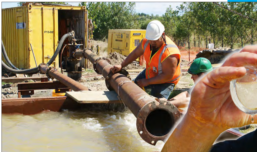
JP MacDonald (left) and Roly Richardson take a close look at the water pouring into the settling tank at 16 litres a second.
