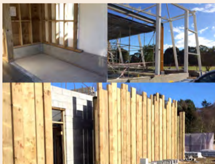
Clockwise from top left: new shower area for sauna users; new framing around the toddlers' pool showing the shape of the building; new palisade fencing around the women's changing room.
