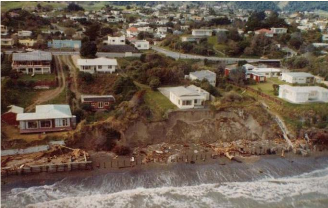
A. Coastal erosion behind failed structures on Rosetta Road following a significant storm in 1976.
