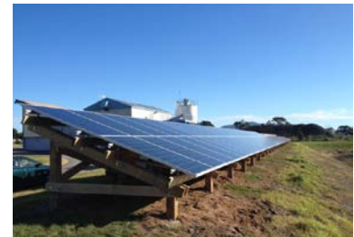
Solar array at wastewater plant
