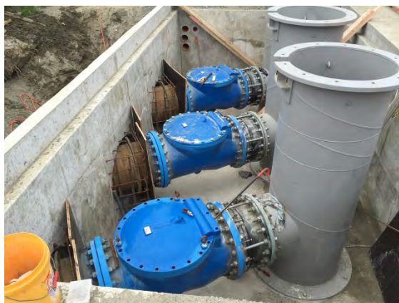
Ōtaki Beach pump station
