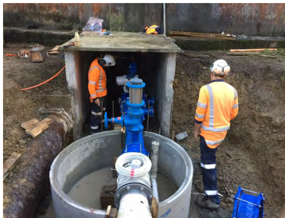
Auto shut-off valve installed at Kākāriki reservoir
