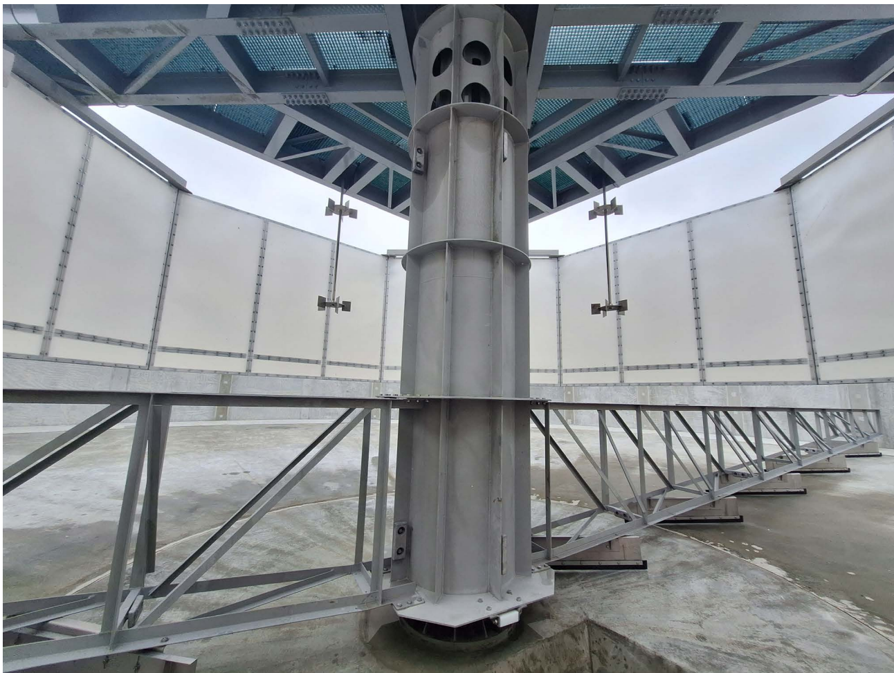
Waikanae Water Treatment Plant clarifier
