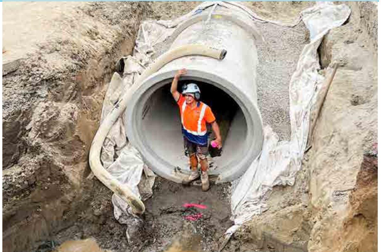
Installation of 800 metres of large diameter stormwater pipe from Iver Trask Place to Amohia Street to reduce flooding issues.
